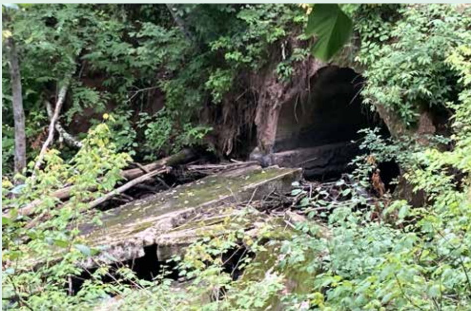
The Nebagamon Creek Railroad Embankment and Culvert Removal Project site. The collapsed culvert, which impedes nearly all fish passage, is visible in the center-right of the photo. Credit: Jeff Tyson, GLFC.
