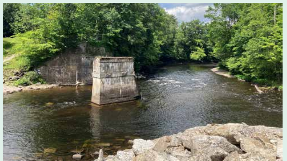
The Salmon River Trestle Pool Project site. The abandoned railroad central pier and left abutment are visible in the center-left of the photo. Credit: Jeff Tyson, GLFC.
